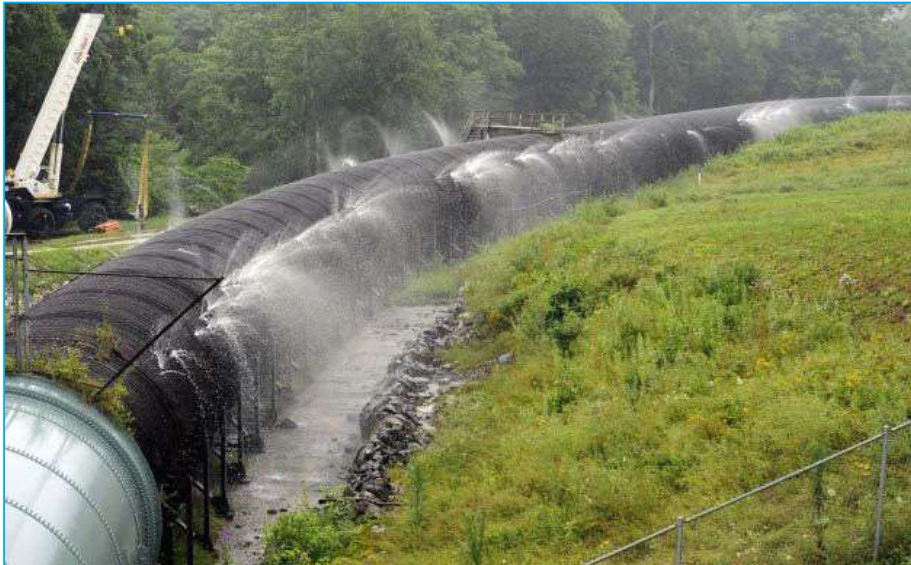
Fig. 16.11: A leaking pipe
