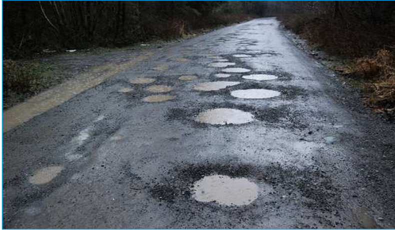
Fig. 16.10: A section of a road with potholes
