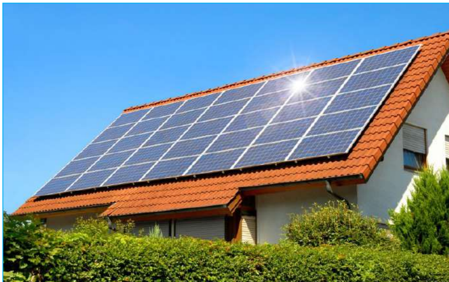
Fig. 14.1: A solar panel on the roof of a house in Sonatube near Kigali City
